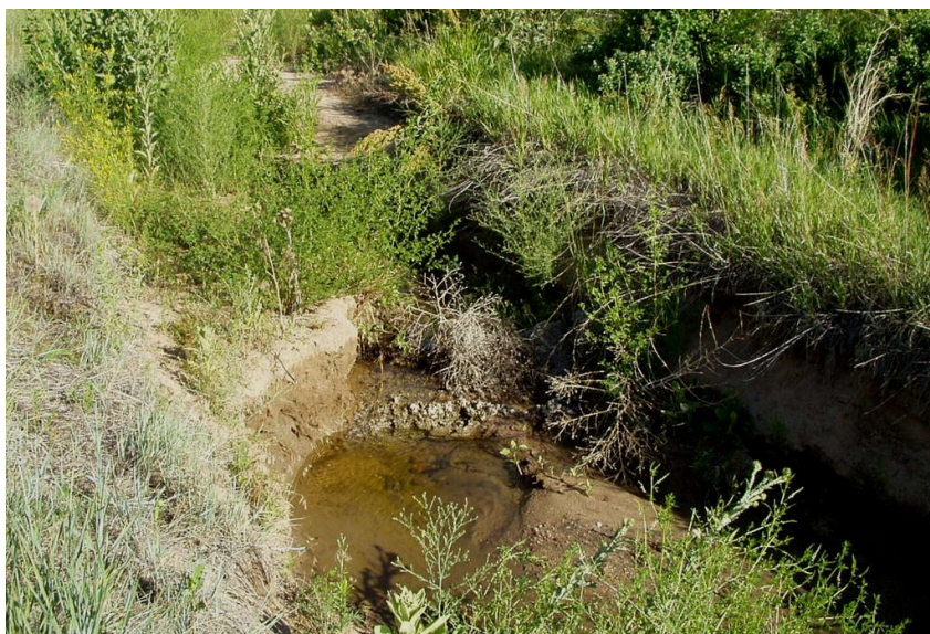
This photo shows the degraded condition of the Upper Marcy Gulch channel before the project.
