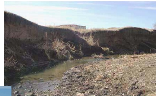
Stream degradation had lowered Cottonwood Creek's channel invert 6 to 8 feet below its historic elevation
