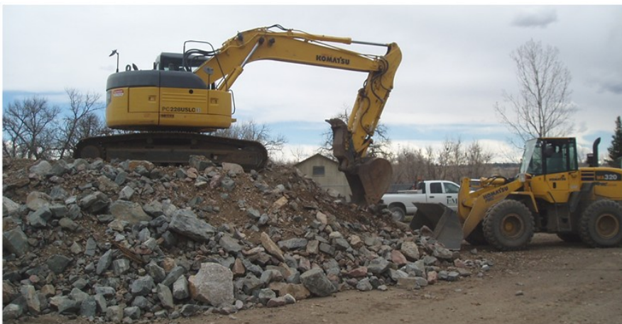
This photo shows void-filled riprap being proportioned and mixed with a loader and excavator.
