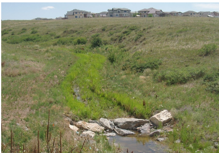
Photo showing boulder drop structure and vegetated void-filled riprap lining beyond.
