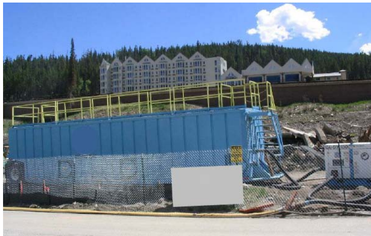
Photograph CT-1. Proprietary chemical treatment system being used on a construction site with sensitive receiving waters. Photo courtesy of WWE.
