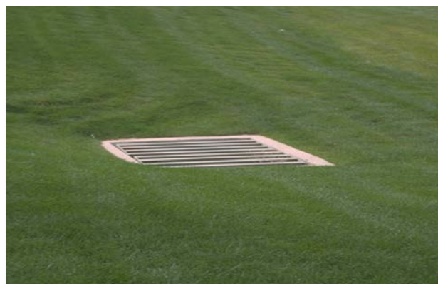
Photograph 7-8. Inlets frequently need maintenance.
