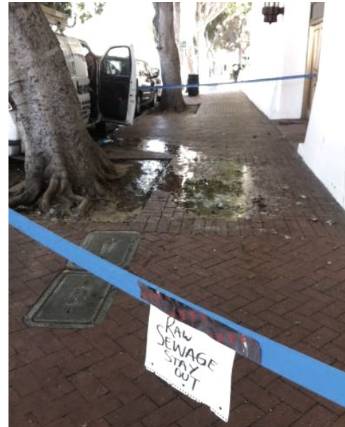
Sanitary sewer overflow. (Photo Courtesy Brandon Steets.)
