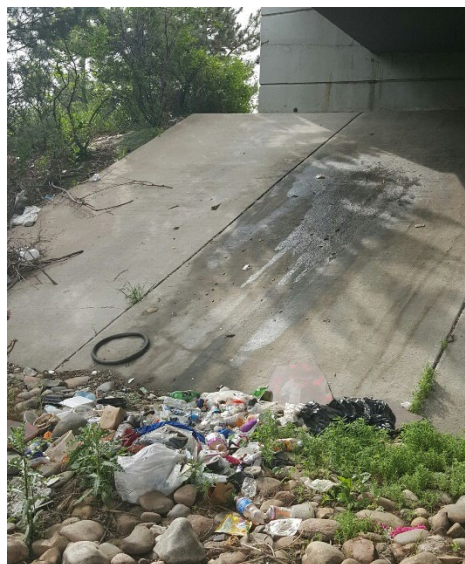
Encampment beneath bridge with human excrement on concrete. (Photo courtesy of Darren Mollendor.)
