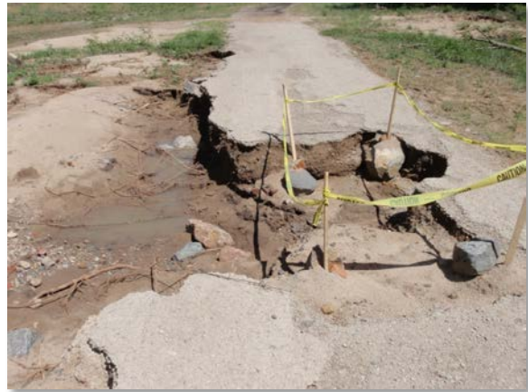
Photograph 10-11. A soil cement path approaching a crossing on Sand Creek is undermined on the downstream side due to overtopping. Overtopping protection was not adequate to stop scour damage before losing a section of the path.
