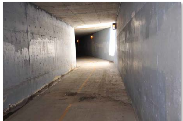
Photograph 10-18. A skylight between C-470 travel lanes brings natural light into the Willow Creek path underpass. Note also sediment deposition on path, typical of a long culvert with a mild slope. Photo courtesy City of Lone Tree.
