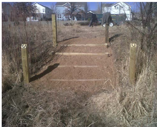
Photograph 10-24. Timber steps filled with roadbase are constructed to provide traction approaching a water crossing. Photo courtesy Arapahoe Park and Recreation District.
