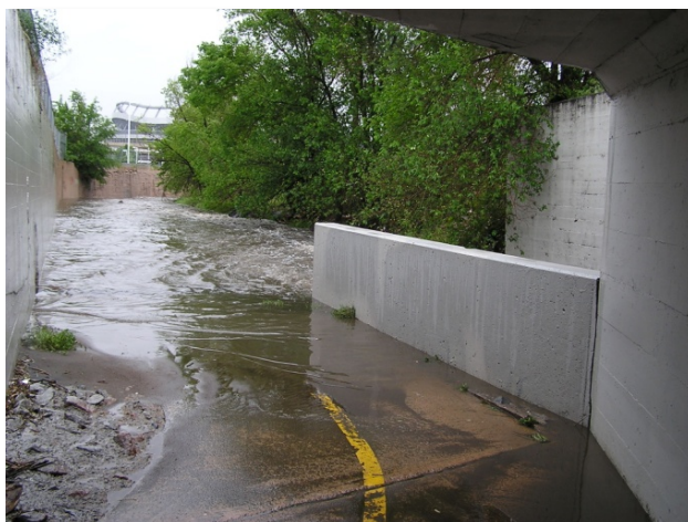
Photograph 10-1. Frequently inundated channels pose a high threat to public safety, especially in a walled channel where water can rise rapidly and egress is limited.
