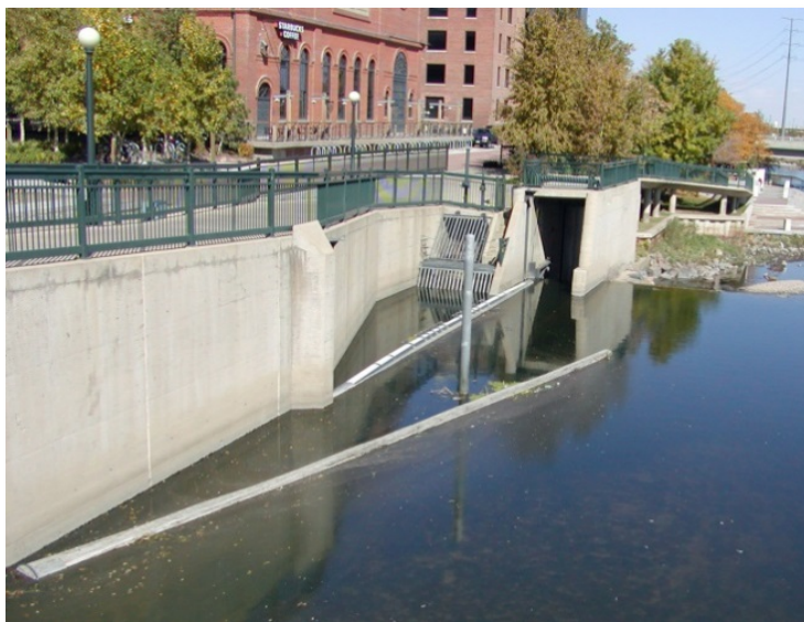
Photograph 10-32. The intake at Confluence Park, Denver is located on the side of the river opposite to where the whitewater bypass is located. In addition to this physical separation, buoys, two debris booms and a bar screen were included to help keep recreationalists away from the intake works. Photo courtesy of McLaughlin Whitewater Design Group.
