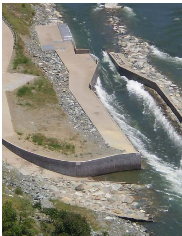
Photograph 10-33. The intake works on the American River near Auburn, California relies on a submerged self-cleaning fine screen. The screen is located in the invert of a boatable channel. This design eliminates intake apparatus that can be hazardous to recreationists, screens for fish and solids, and has proven to require relatively little maintenance. Photo courtesy of Placer County Water Agency.
