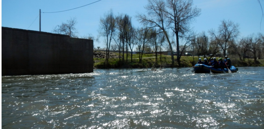
Photograph 10-39. The “pier nose extensions” on this bridge reduce the accumulation of debris and thereby improve safety for in-river users. Photo courtesy of McLaughlin Whitewater Design Group.
