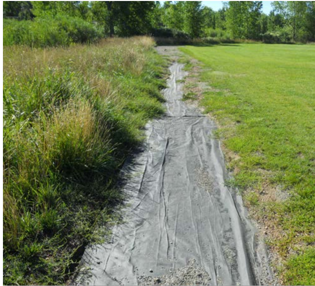
Photograph 10-27. Geotextile is all that is left of this crusher fines trail that washed out on Goldsmith Gulch.
