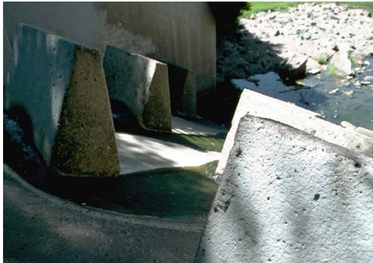
Photograph 12-3. Baffle chute drop after several decades of service.
