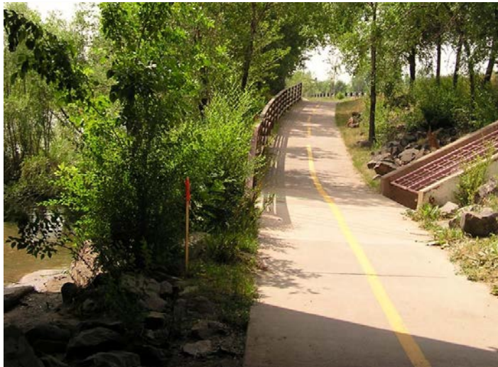
Photograph 10-10. Along this section of the South Platte River, the combination of a steep longitudinal slope, a cross drainage structure, and a steep slope from the path to the water warranted both a safety rail and striping.
