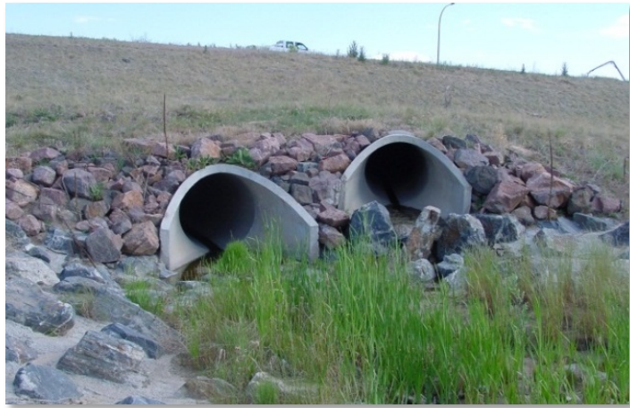
Photograph 11-4. Energy dissipation and outlet protection are essential to promote channel stability.
