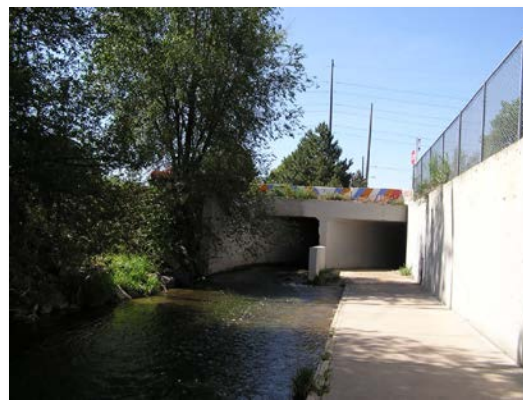
Photograph 10-16. Multi-cell culverts can be uninviting, especially if the user is not able to see the other end.
