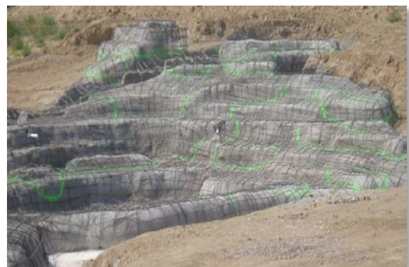
Photograph 9-26. Spray paint is used on the “skim coat” of a sculpted concrete structure prior to concrete placement to identify the locations for fracture lines and other features.
