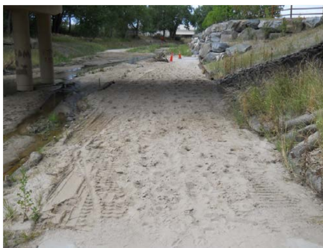
Photograph 10-2. Sediment frequently accumulates under crossings. Frequently inundated paths collect sediment and are maintenance-intensive.
