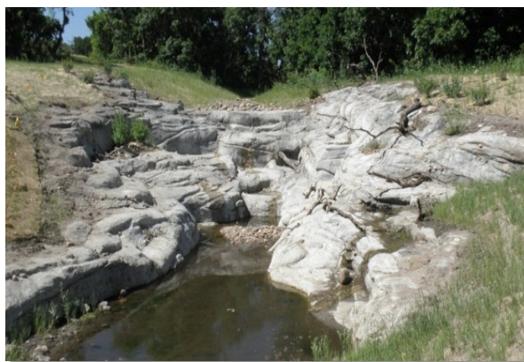
Photograph 9-10. This drop structure located along Oak Hills Tributary represents a complex design example.
