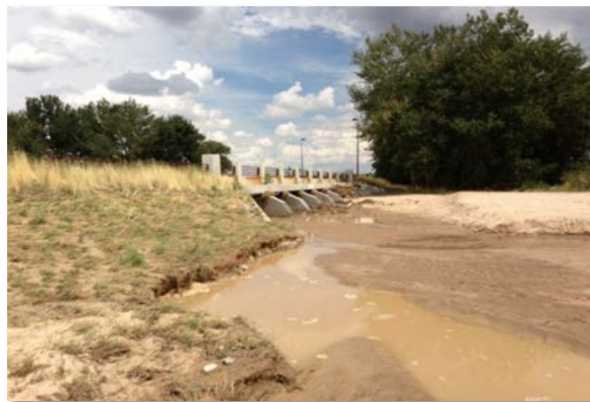
Photograph 11-2. Culverts at a skew can be sediment traps. Where they cannot be avoided consider how the design can best facilitate maintenance including sediment removal.
