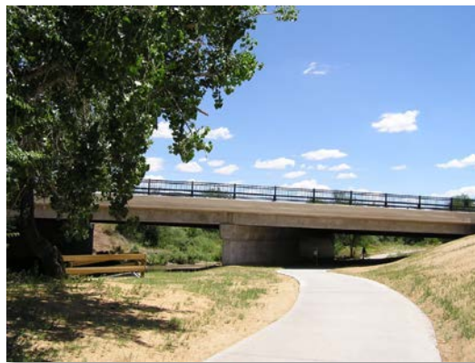
Photograph 10-14. This bridge offers safe passage, providing the user with a view of potentially rising water and the path beyond the structure. Additionally, the slope from the path to the roadway offers the user a passable route to higher ground in case of flash flooding.
