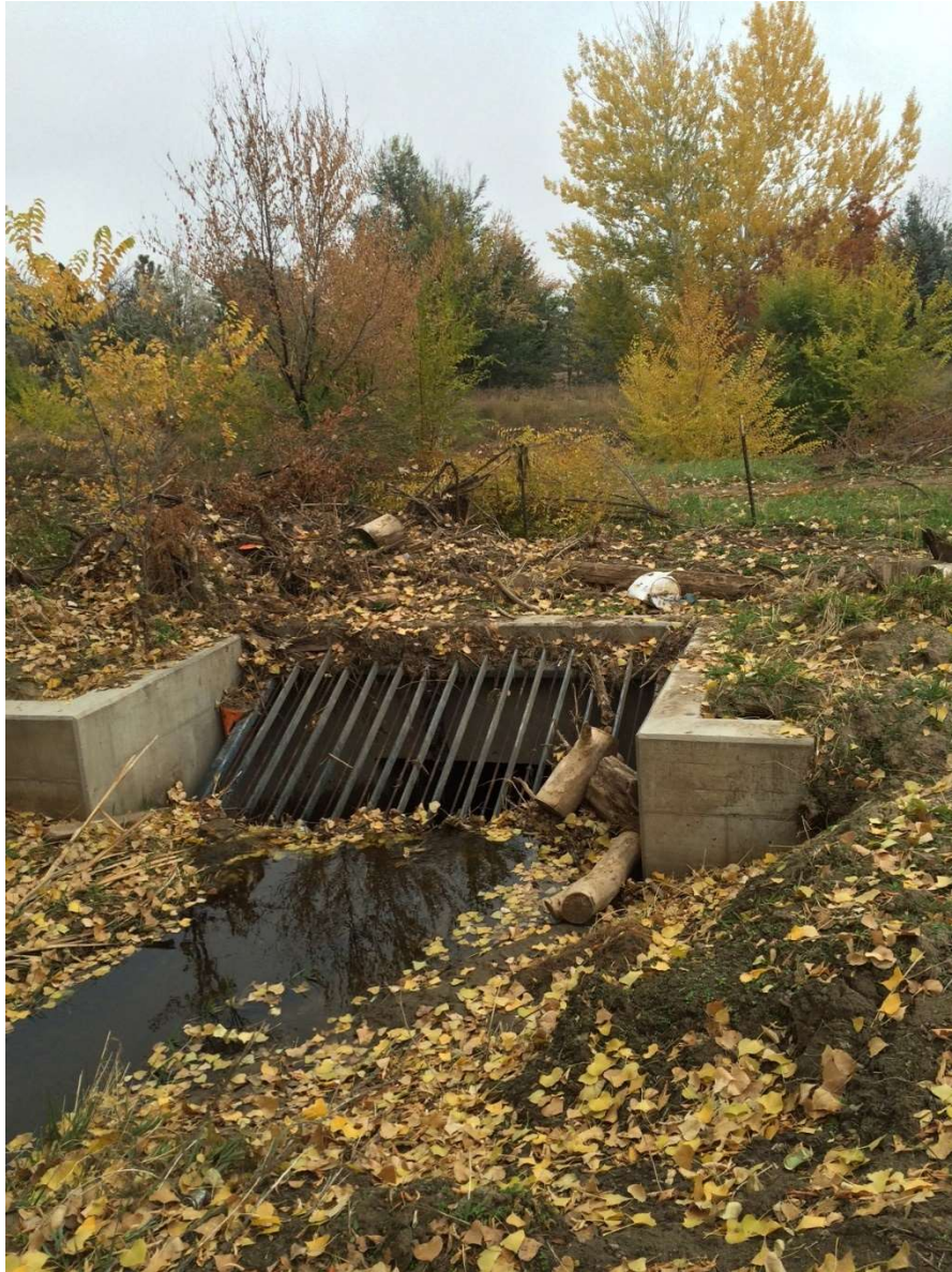
Figure 7. Van Bibber Creek is conveyed under the Croke Canal upstream of 320 Sports Complex
