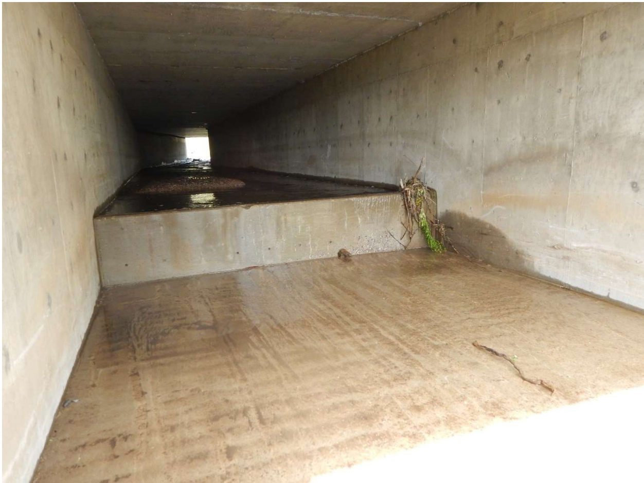
Figure 4. Photograph of the diversion wall inside the reconstructed culvert downstream of gage 330 at Hwy 93.
