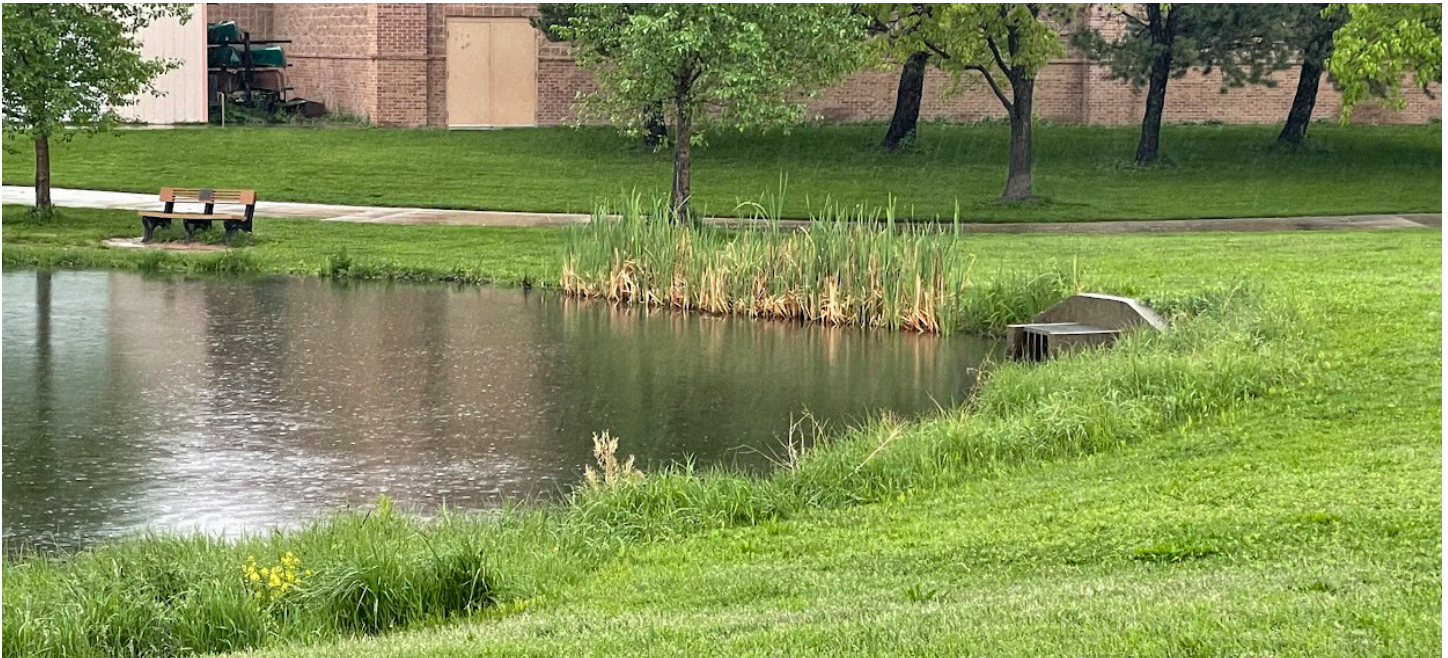
Photograph 4-19. Retention pond outlet structure blends with the bank and is easily accessible for maintenance.
