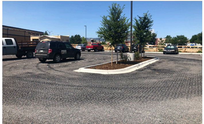
Photograph PPS-17. PGP parking area with markers to delineate parking spaces. Photo: True Grid
