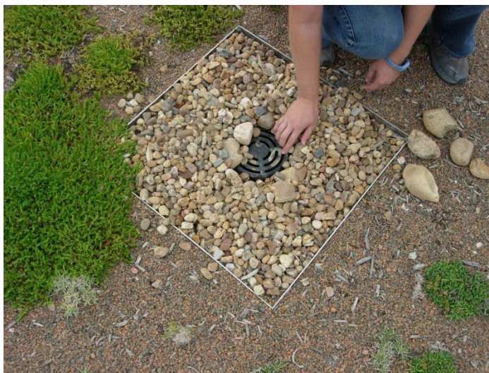
Photograph 6-3. When inspecting roof drains, remove any surrounding rock as well as the inlet grate and visually inspect the drainpipe to ensure it is free of any extraneous materials.
