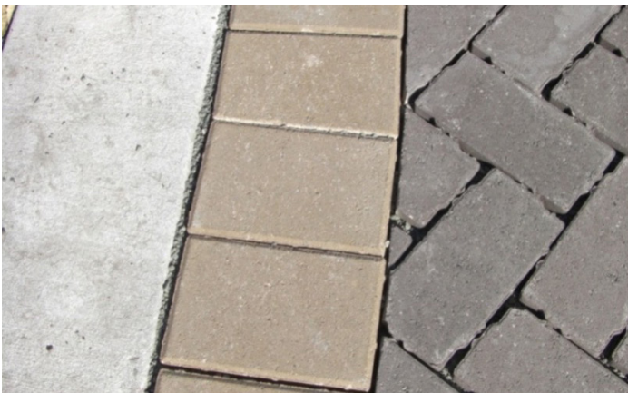
Photograph PPS-14. The very small cut paver shown in this photo could have been eliminated by rotating the paver above it 90 degrees.
