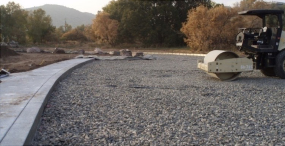
Photograph PPS-9. The reservoir layer of a permeable pavement provides storage volume for the WQCV. Photo: Muller Engineering and Jefferson County Open Space.
