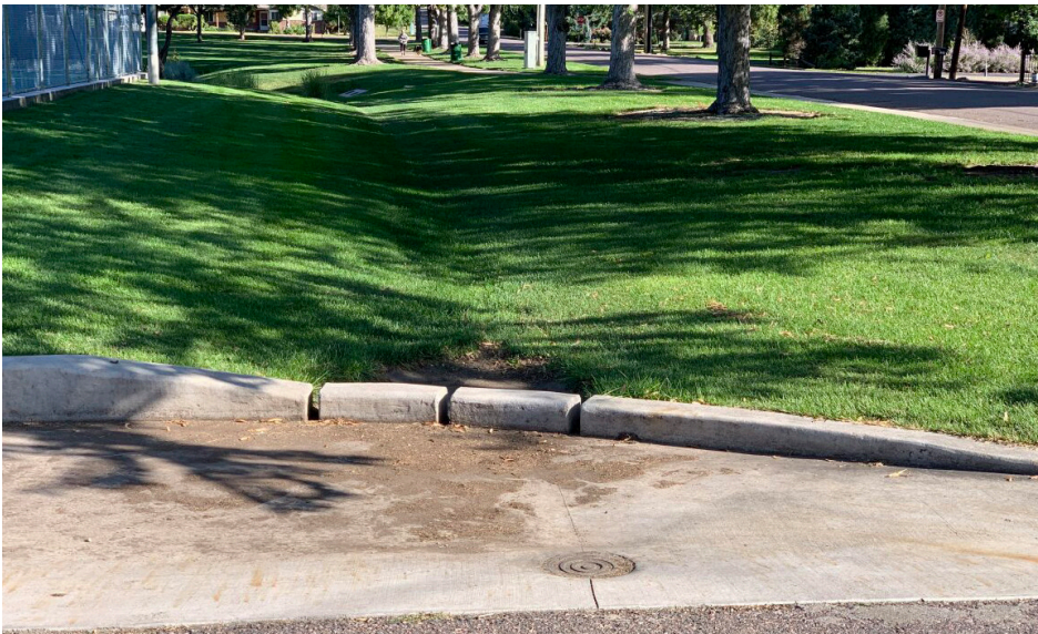
Photograph RPA-10. Sediment forebay at the entrance to a grass swale leading to an EDB concentrates maintenance needs at entrance of swale. This is an example of a three-step treatment train: forebay, swale, pond.
