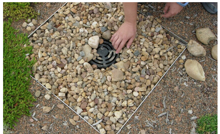
Photograph GR-5. Metal edging separates substrate from rock that surrounds the roof drain. It also serves to facilitate regular maintenance by limiting plant and root growth near the drain.
