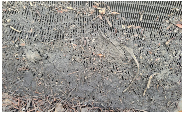
Photograph EDB-5. Well screen is intended to protect small orifices from clogging; however, the fine screen is itself subject to clogging and requires frequent inspection and maintenance to keep clear.
