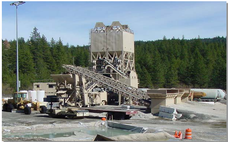
Photograph TBP-1. Effective stormwater management at temporary batch plants requires implementation of multiple BMPs. Photo courtesy of California Stormwater BMP Handbook.
