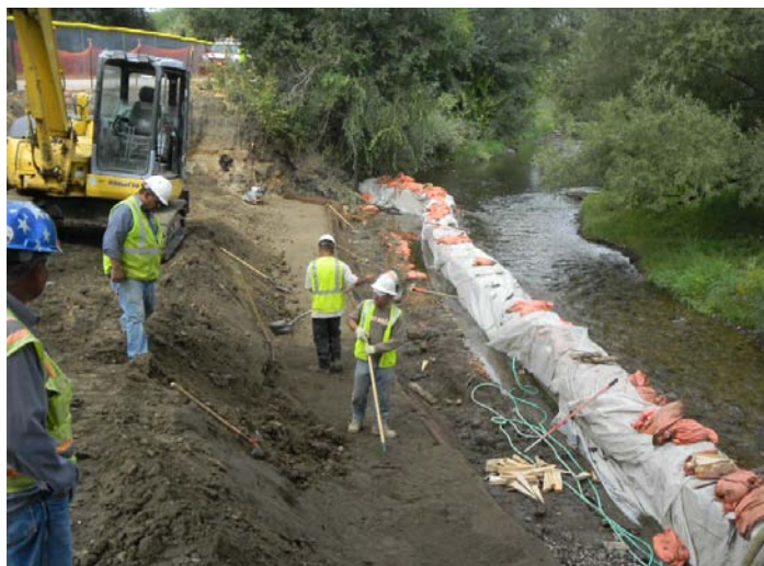
Photograph TDM-1. This coffer dam, installed to allow grading and stabilization of the stream bank, consists of concrete blocks covered by an impermeable liner held in place by sand bags.
