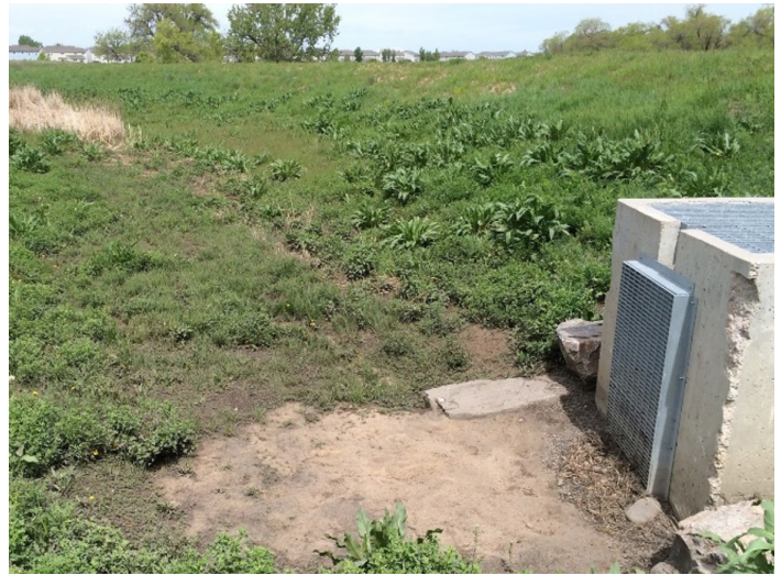
Photograph EDB-7. This EDB was originally constructed without a micropool and was retrofitted with a sand filter with underdrain to reduce the potential for clogging the outlet and water backing up in the basin.
