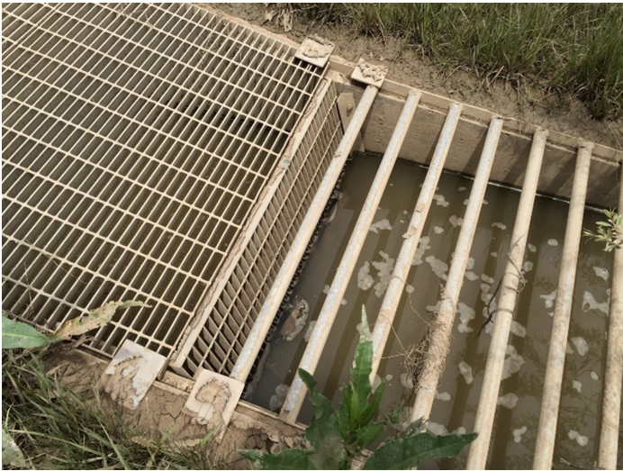
Photograph EDB-6. In this outlet, runoff flows through safety grating (5-inch clear bars) to separate floating debris before continuing through standard bar grating that extends to the bottom of the micropool. The grating extending down into the micropool can be raked through the gap in coarse safety grate to clear debris.
