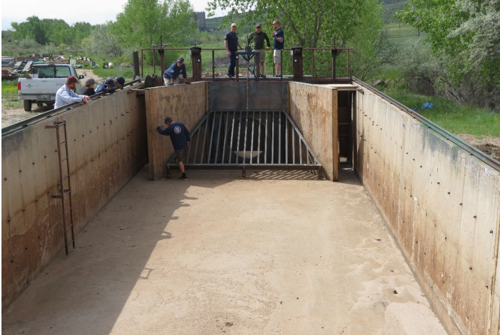
Figure 1. A View of the 20-foot Flume Fitted with a Grate and Wing Walls
