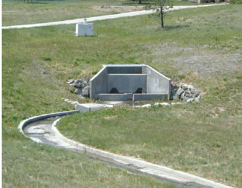
Photograph 3. Energy dissipater, forebay, and trickle channel
