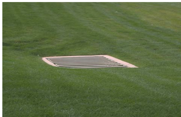
Photograph 7-8. Inlets frequently need maintenance.
