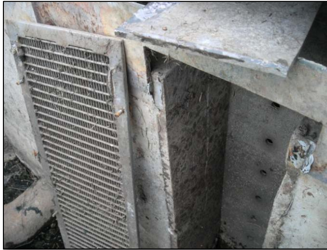
Figure 1. The current standard for water quality outlet design includes a column of small orifices, protected from clogging by a well screen (shown removed for maintenance). The well screen was added after earlier installations demonstrated a great propensity for clogging. Unfortunately, the well screen also becomes clogged and is considered a significant maintenance issue for CDOT field personnel.
