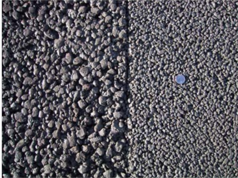
Photograph 2. The installation included two mixes utilizing different aggregate. The AASHTO #67 mix is shown left, AASHTO #8 shown right.
