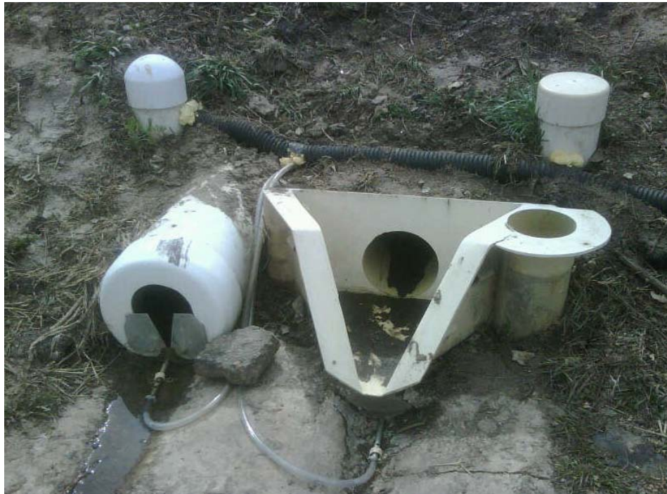
Photograph 4. The V-notch weir for the pervious concrete (left), and the H-flume weir for the reference site (right), with stilling wells in the background.
