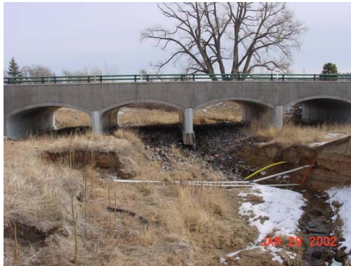
Figure 2. Stream degradation and erosion in Denver, USA area. Note the 2- to 3-meter incision, exposed utilities and head cutting that is undermining the bridge pier.
